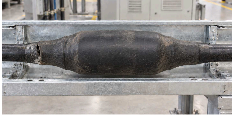
BEFORE: JOINT SEAL নষ্ট
