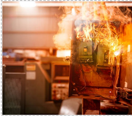
AFTER THE DISCHARGE burnt panel internals · charred wiring
