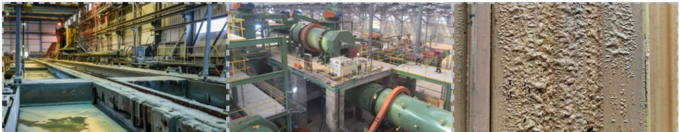
Acid fume attack — pickling shed
