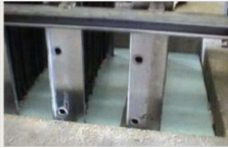
FM-71 mortar seal — cable tray through shear wall
