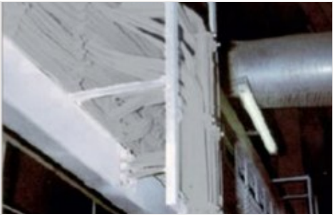
EC 43 coated cable bundle — after fire test
