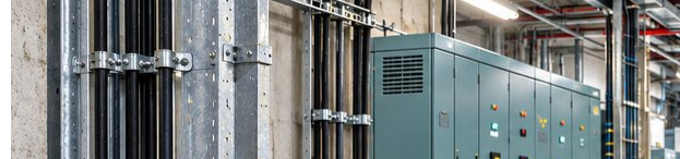
EC 43 General · Cable runs
