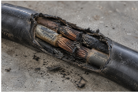
INSULATION FAILS. CONDUCTORS SHORT. CIRCUITS FAIL.
