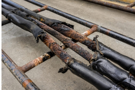
BURNT CABLES. COSTLY REPLACEMENT. COSTLIER SHUTDOWN.
