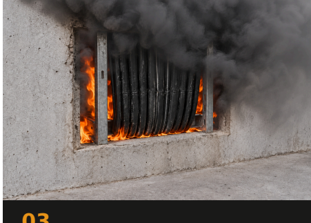
03 FIRE + SMOKE CROSS UNSEALED OPENINGS
