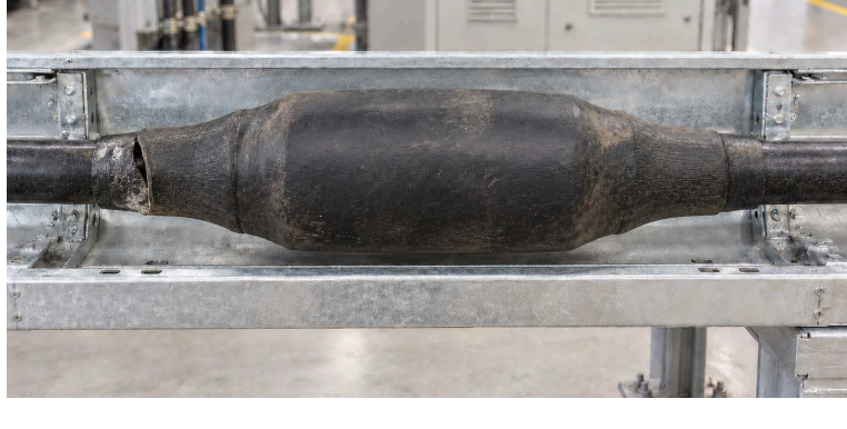
BEFORE: JOINT SEAL ଖରାପ
