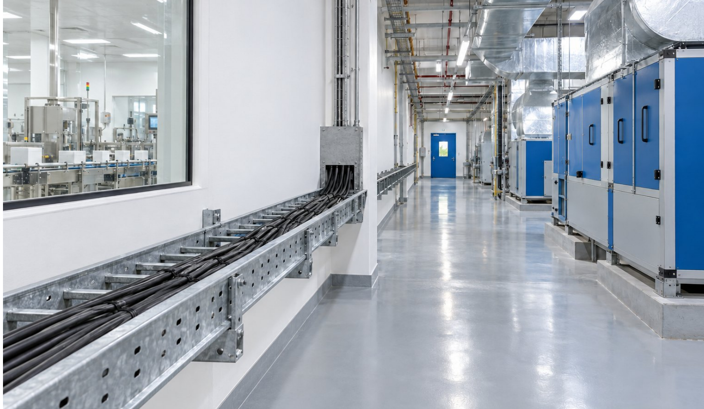
AHU service gallery and cable route.
