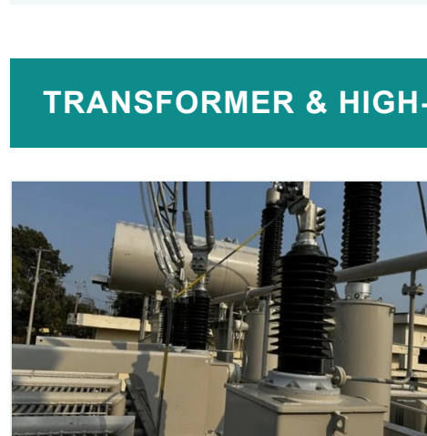
A leaking transformer sealed without shutdown.
