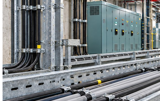
EC 43 General · Cable runs
