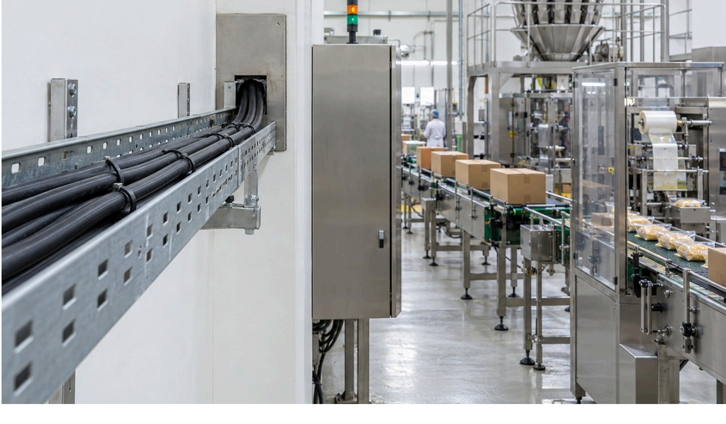
Packing-line cable entry.
