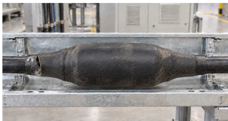
پہلے: JOINT SEAL خراب
