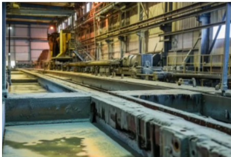
Acid fume attack — pickling shed
