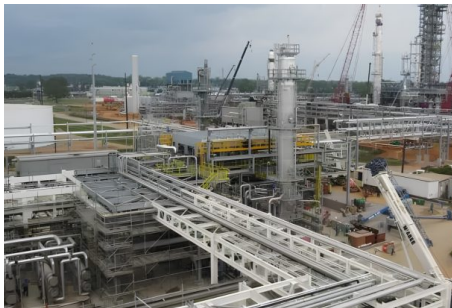
Rusted live-unit steel — blasting impossible
