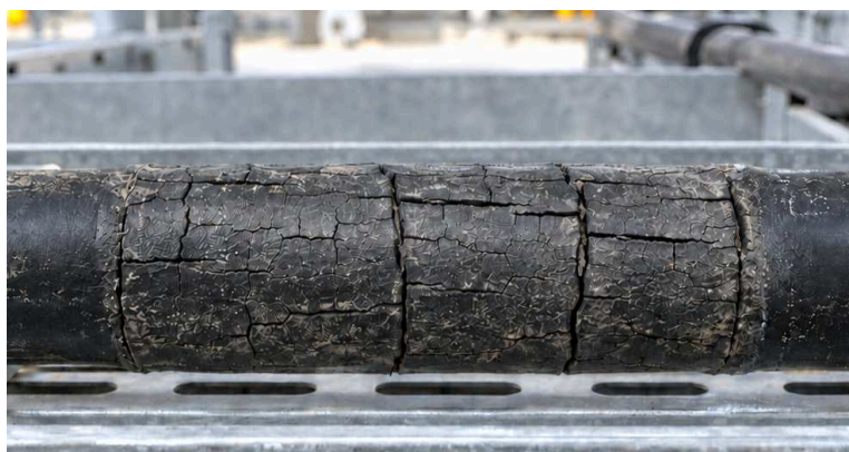
BEFORE: CRACKED SHEATH
