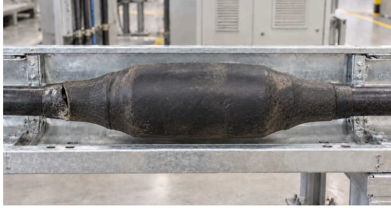
BEFORE: FAILED JOINT SEAL
