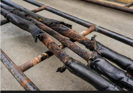
BURNT CABLES. COSTLY REPLACEMENT. COSTLIER SHUTDOWN.
