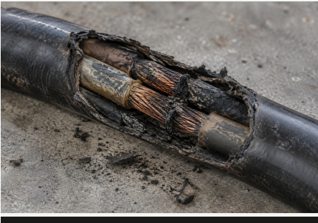
INSULATION FAILS. CONDUCTORS SHORT. CIRCUITS FAIL.
