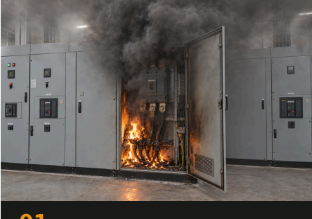
01 PANEL CATCHES FIRE. SMOKE BUILDS.
